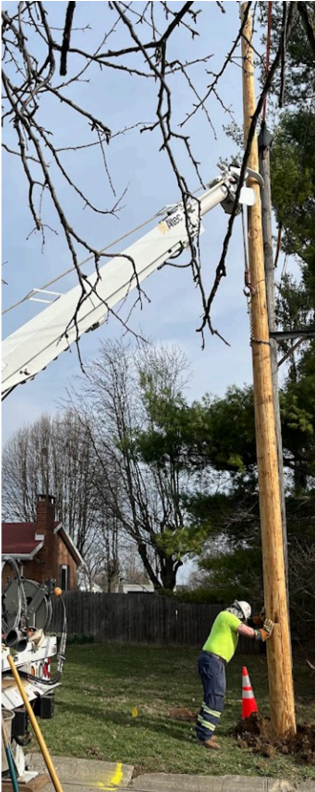
Recent electric and metering projects.
